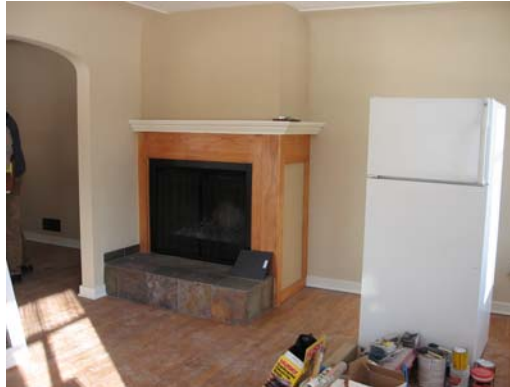
Fireplace in Living room Replaced faux stone paneling with slate base and wood trim.
